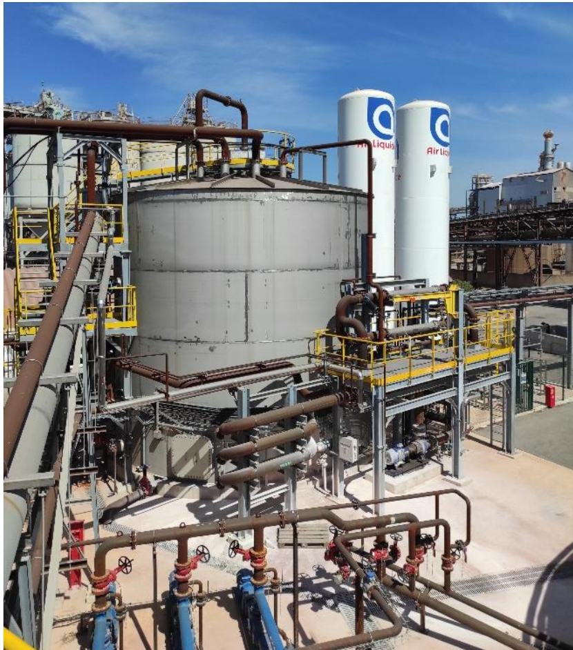
Figure 9. CO 2 neutralization plant.
