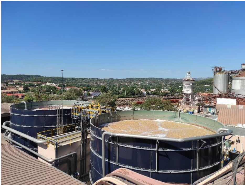
Figure 10. Biological treatment plant.
